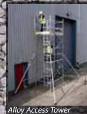
Alloy Access Tower
